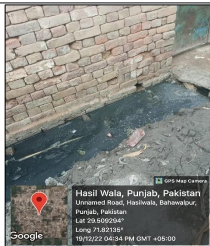
Clogged sewerage channels
