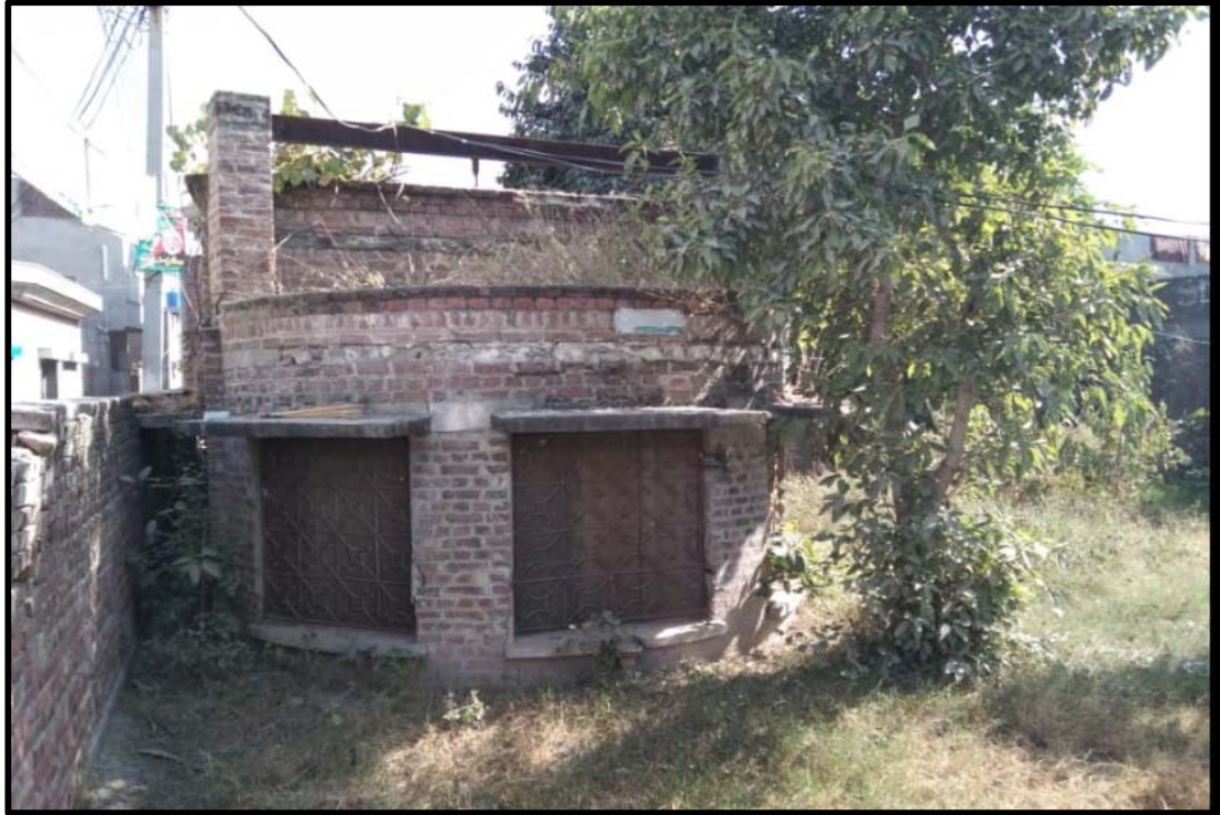
Proposed site for installation of S/AC filter with fluorination in village dhokal
