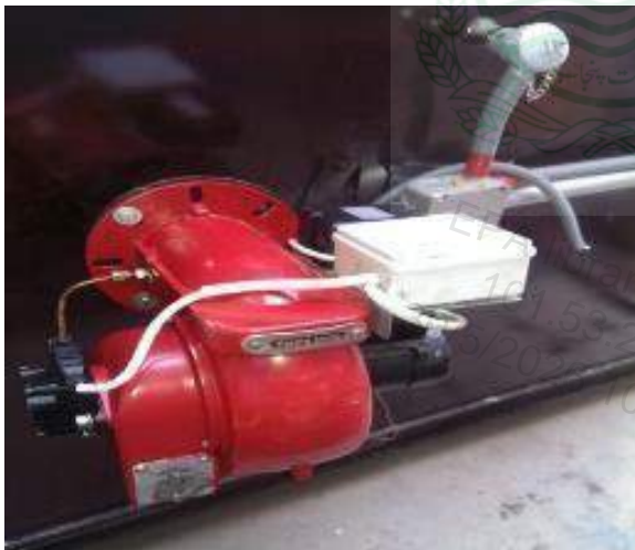
Figure 3-5: View of Burner
