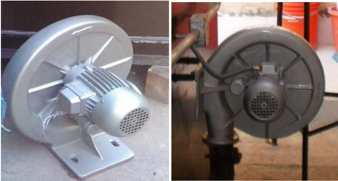
Figure 3-6: View of Air Supply Fans
