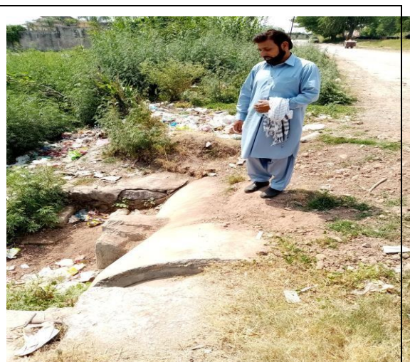
Another above ground part of conductance main
