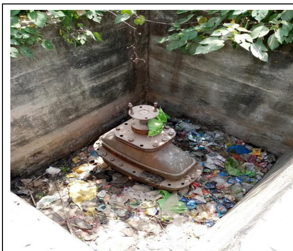
Valve chamber at conductance main
