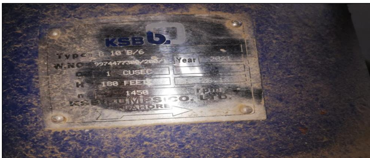
Figure 6-14, KSB Pump Installed in Shallow Tubewells Installed Under PCP Showing Discharge 01 Cusec
