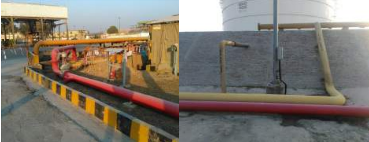
Figure 4-9 Fire Water Tank Pipelines
