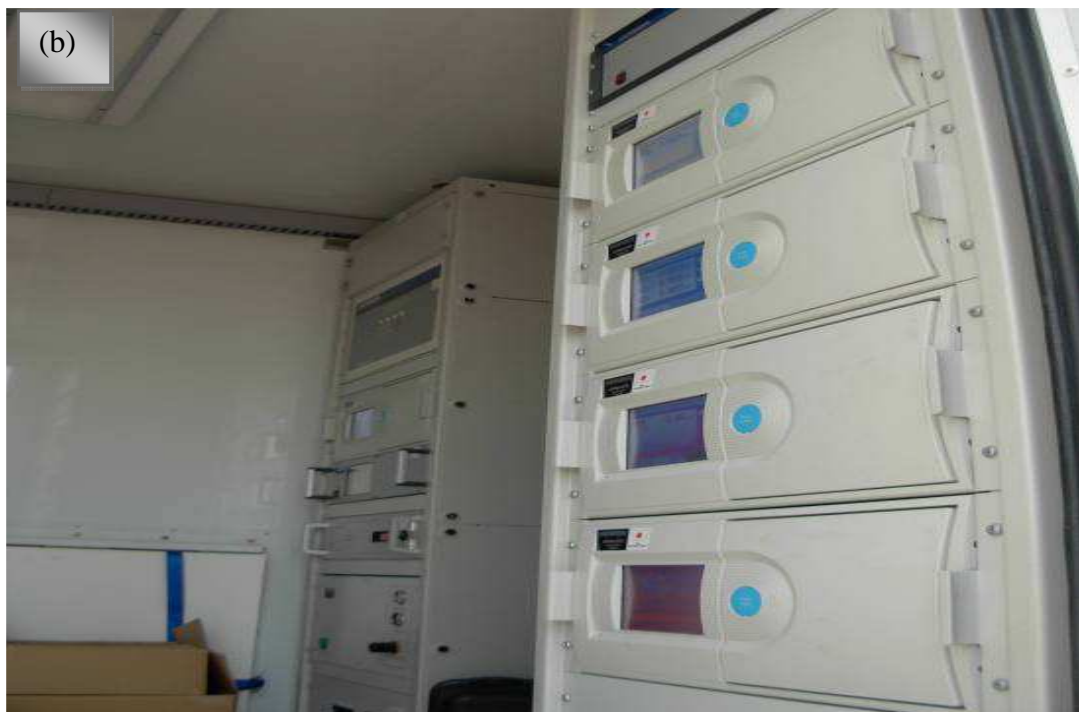
Fig. 3.2.a. Air quality monitoring station (a) mobile station and (b) analyzers
