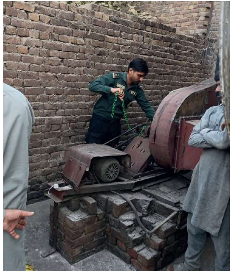
Sealing of Industry Boiler
