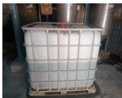
Chrome Recovery Plant
