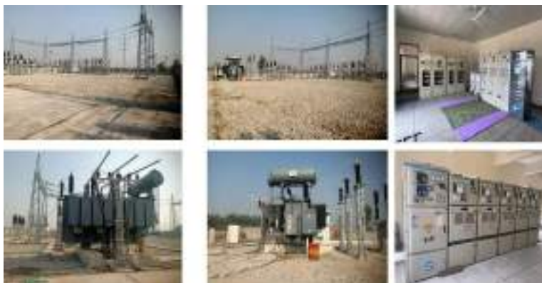
132 KV STZ Grid Station
