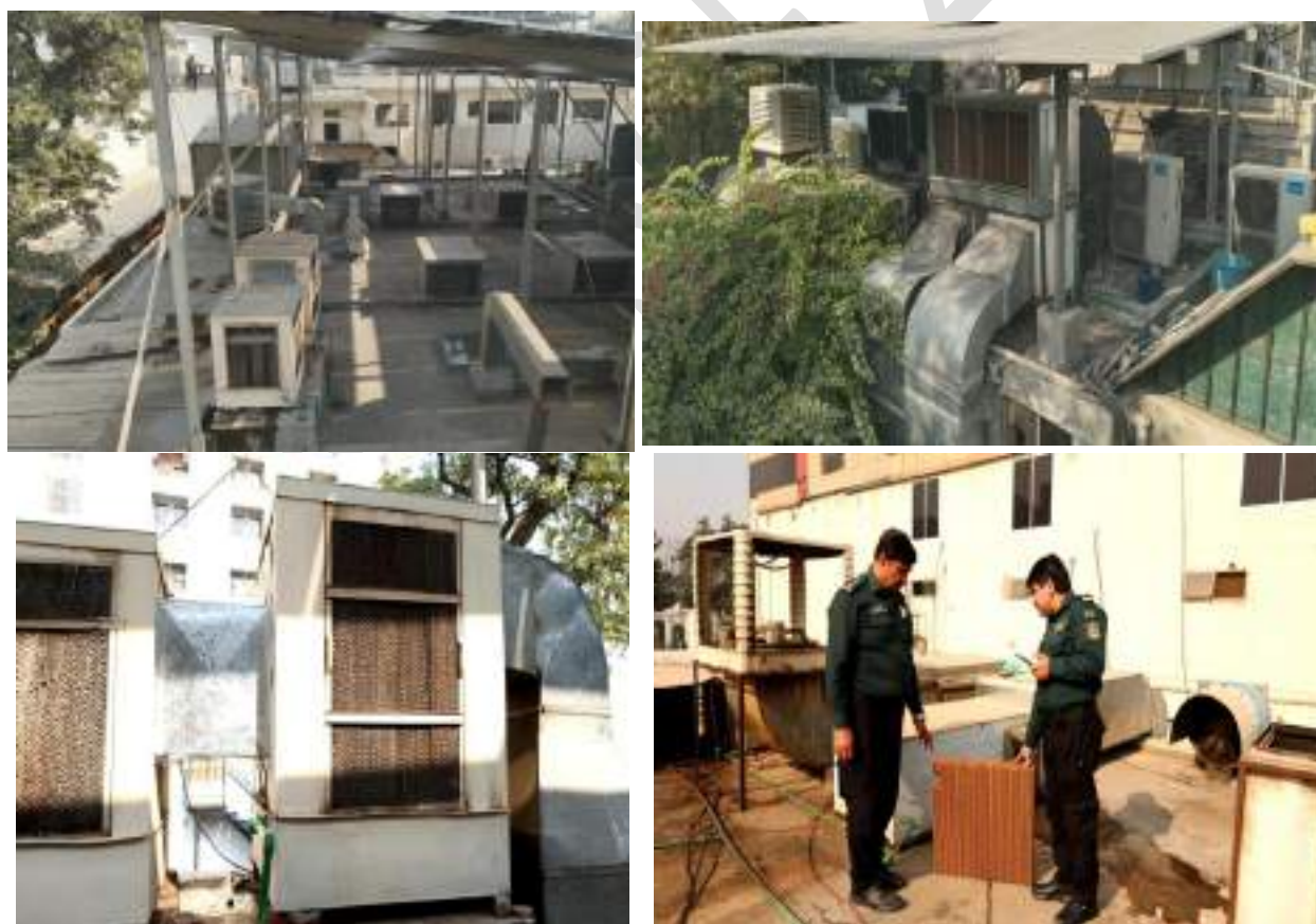
Figure 5.24: Installation of Suction Hoods at Restaurant
